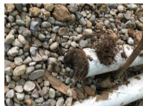
Roots in pipes
