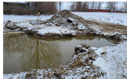
Winter installation that is not going well.
